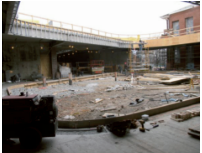
Courtyard in progress. Slated for glass curtain walls and open to the sky, this space will one day hold landscaping and provide natural light to the surrounding commons area. A rolling glass door will be installed on the far side.
