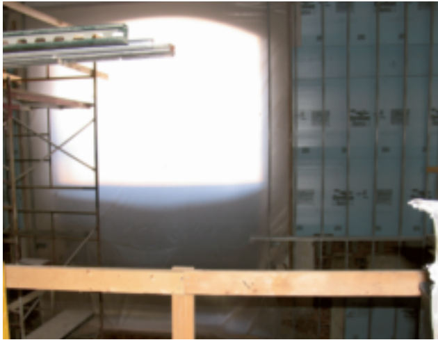
View of picture window space in Trickett Hall. A new staircase will be built below.
